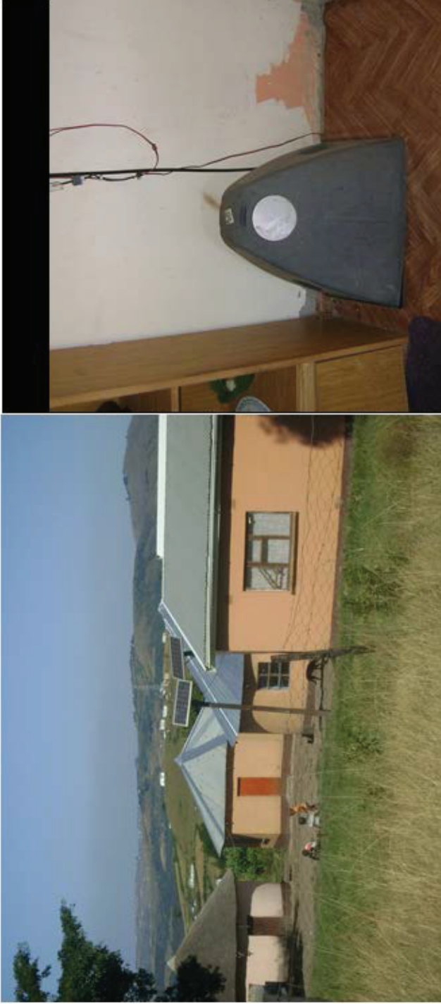
Figure 6.2: A home with SHs (left); a malfunctioning battery storage unit which the households cannot repair (right) Source: Pictures taken during fieldwork by the author
